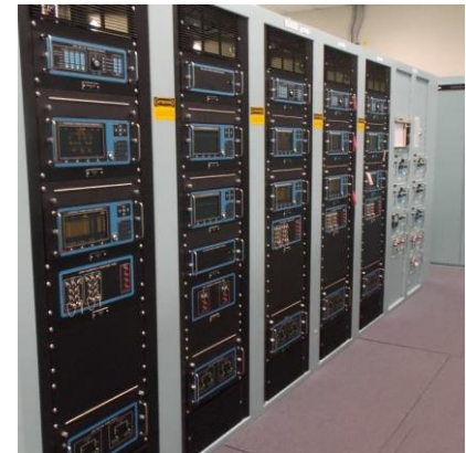
Digital Power Range Monitoring (Columbia)
