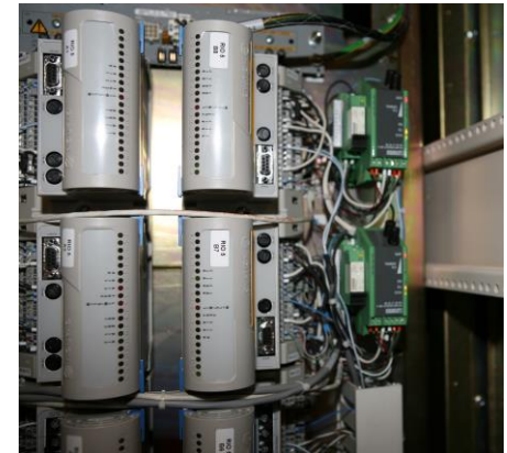
Distributed Control System (McGuire)
