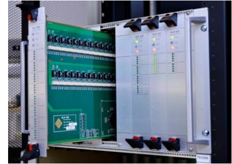
Digital Reactor Protection System (Diablo Canyon)
