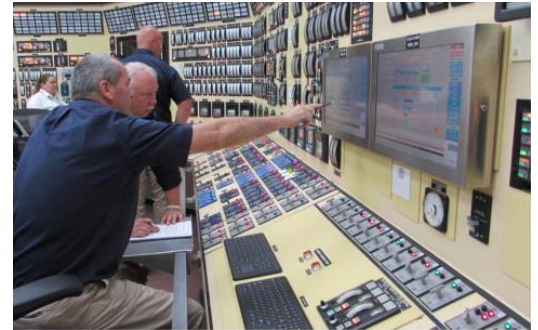
Turbine Control Upgrade (Vogtle)
